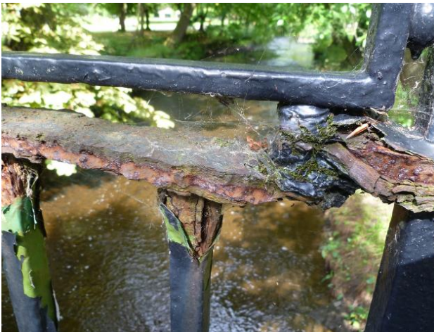
Corrosion of lower bridge parapet prior to restoration
