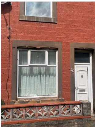
Front elevation requiring repainting
