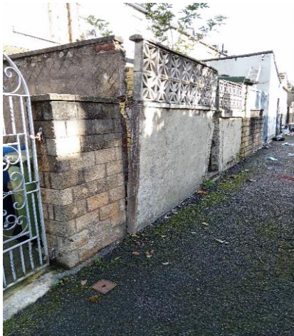
Dangerous yard wall
