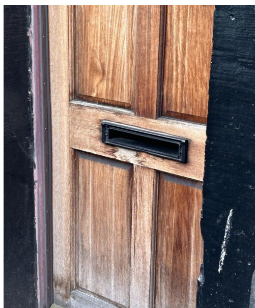
Property with no letter box cover and in poor condition
